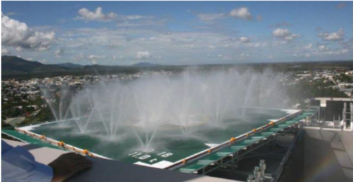
Figure 16-6: A water-only DIFFS on a heliport with a passive fire-retarding surface
