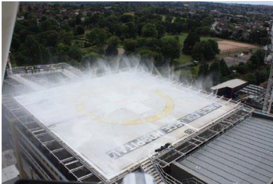
Figure 8-5 – A foam DIFFS on a solid plate surface at an elevated heliport
